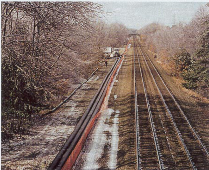
DURING CONSTRUCTION, as many as three 18 in. (457 mm) polyethylene pipes were used to reroute the sewage flow in some of the sections being rehabilitated.
