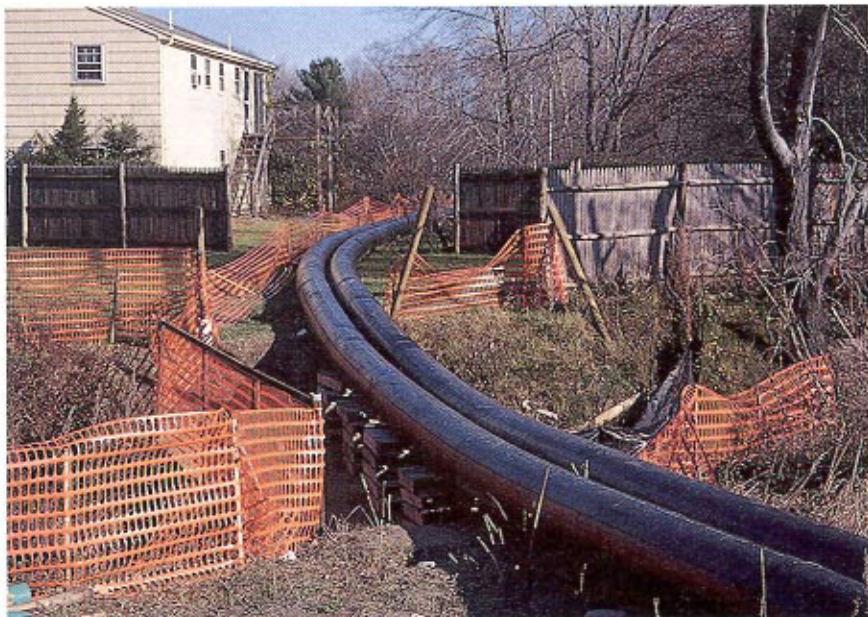
BECAUSE THE pipeline runs through such sensitive areas as wetlands and even residential neighborhoods, the MWRA decided to avoid open-trench excavation.
