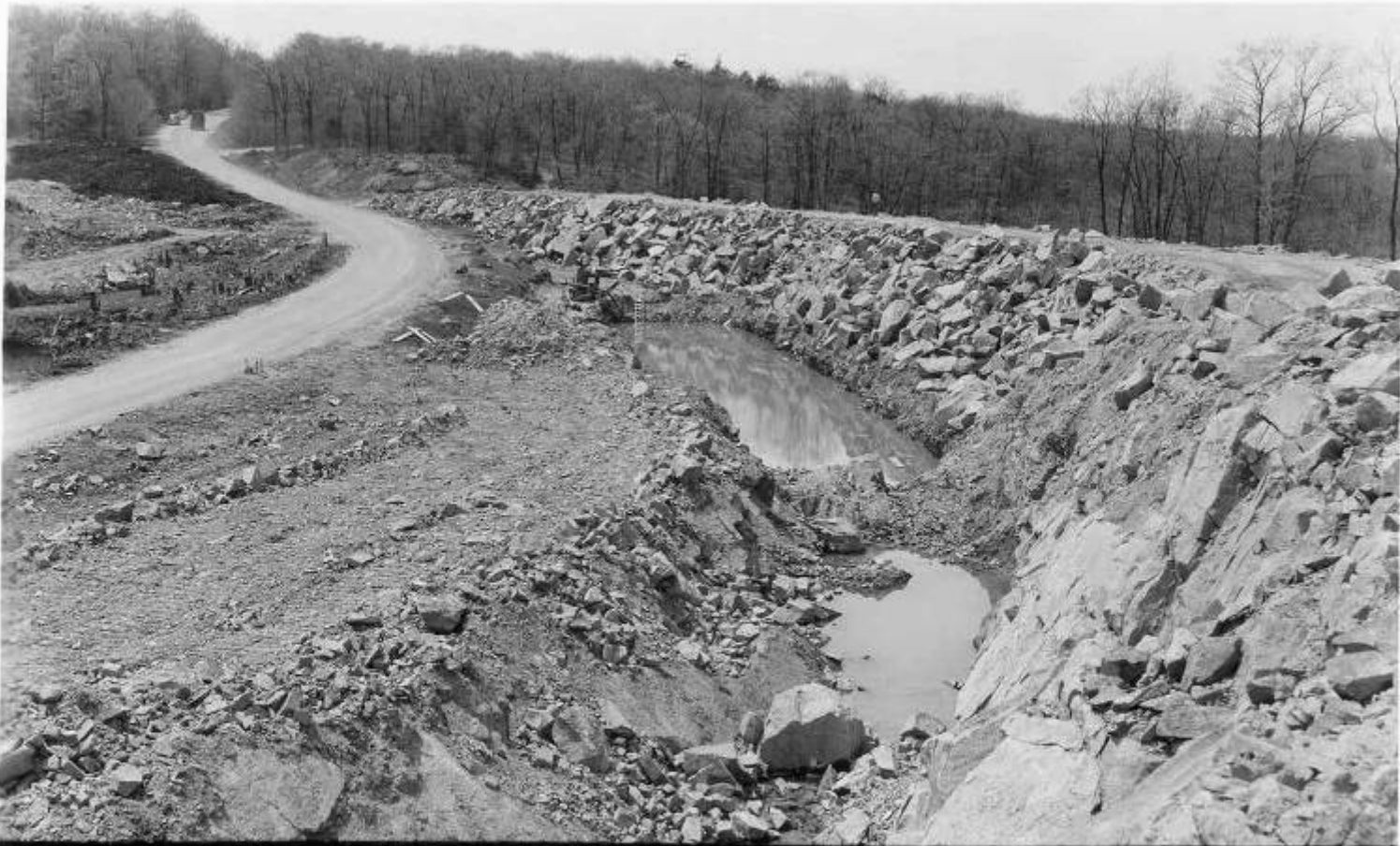
Looking W'ly from Highway Sta. 10+50 showing excavation for core wall footing Blue Hills Reservoir - Cont. 187 - 5/12/50 - Photo Maley 187 - 53
