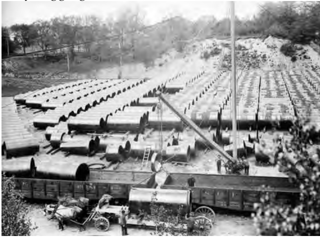
Trans-loading cast iron pipe from rail to horse drawn carriage for delivery
