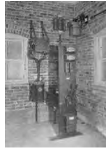
1923 Pump control panel
