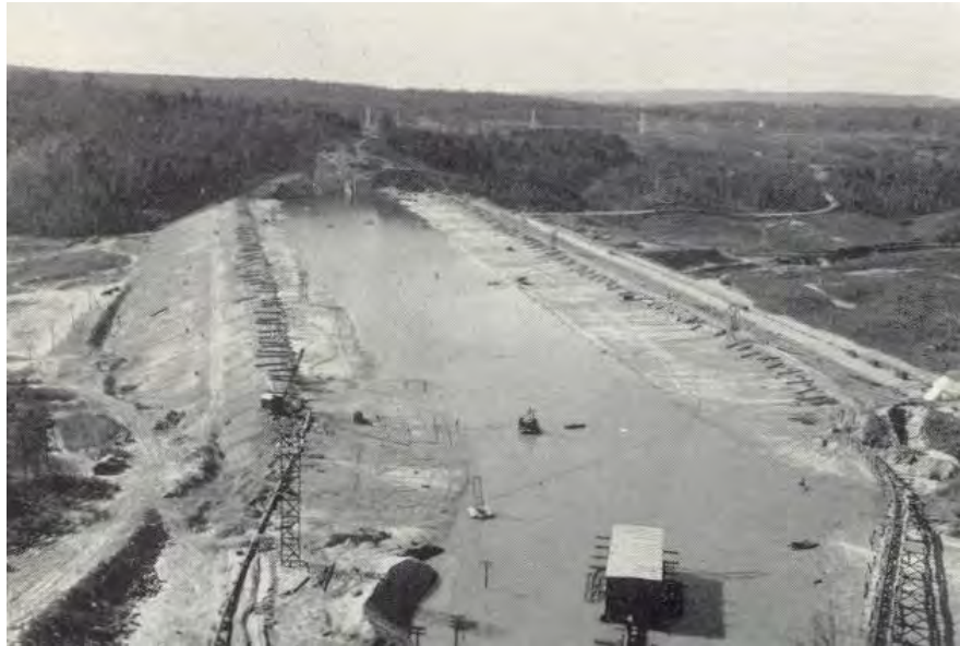
Construction of hydraulic fill Winsor Dam at Quabbin Reservoir, MA – Note that the Dam is named for Frank Winsor who also built the Gainer Dam for Providence
