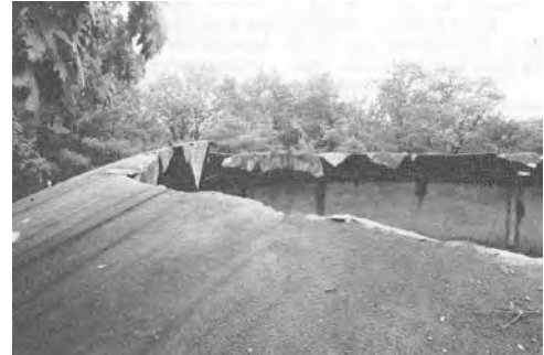
1988 Holden MA dome failure
