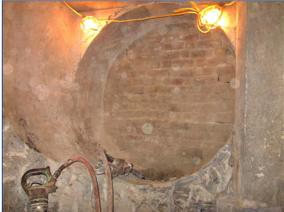
Demolition activity within the existing Boston junction chamber to connect the 54-inch Brookline Connection pipe to the 108-inch South Charles Relief Sewer.
