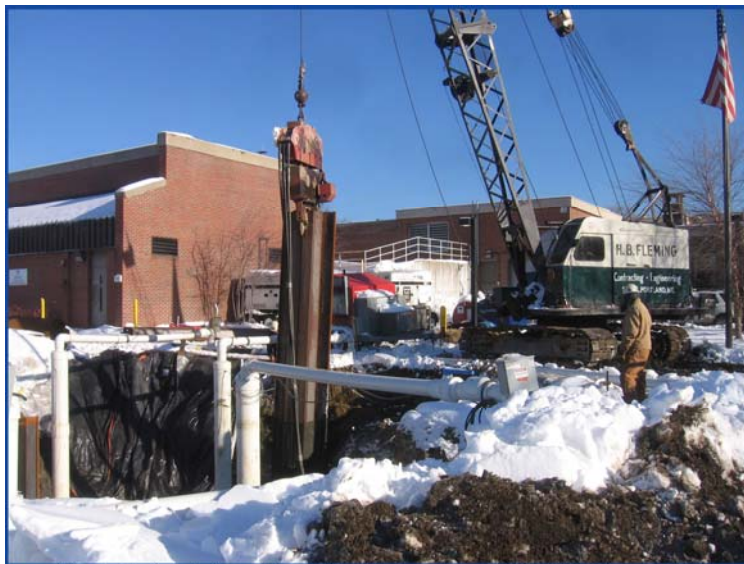
Sheet pile installation at Cambridge Cottage Farm CSO facility for new PCCP pipe interconnection between the North and South Overflow Chambers.
