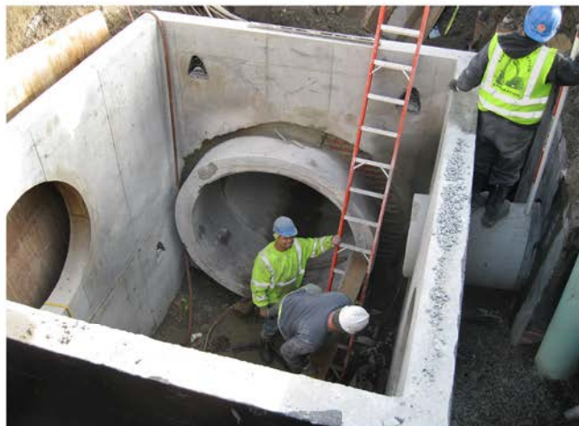
Installation of Special Manhole C at West First Street and F Street
