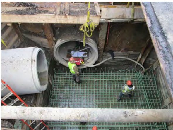
Special Manhole B at E. First St. and K St. (Contract 3B)
