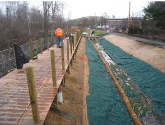
Construction of Boardwalk and Vegetated Swale from Forebay to Main Wetland Basin, December 2012
