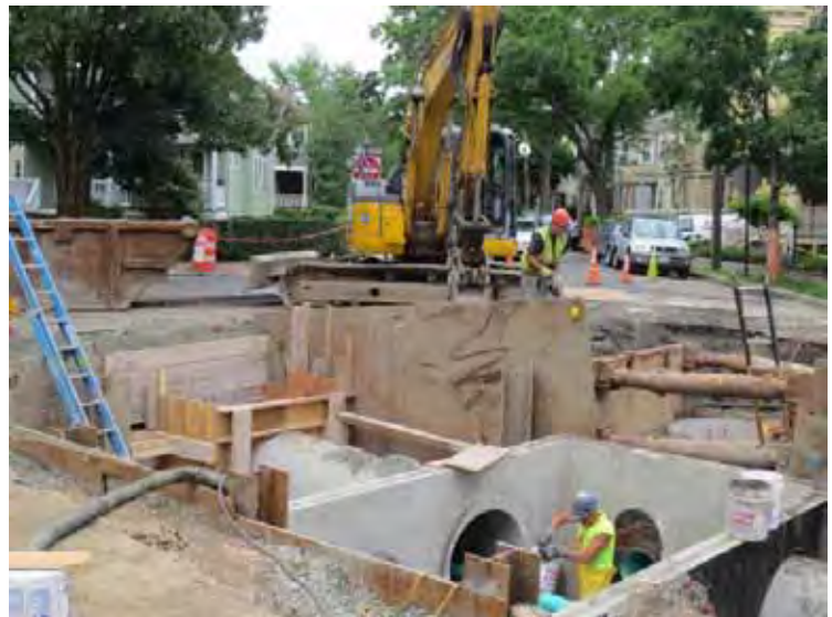
Installation of Drain Vault #1, Vassal Lane and Standish Street, CAM004 Sewer Separation Contract 8A
