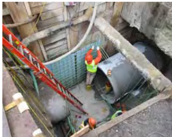
Construction of drain manhole at K and E. 2 nd streets Reserved Channel Contract 3B
