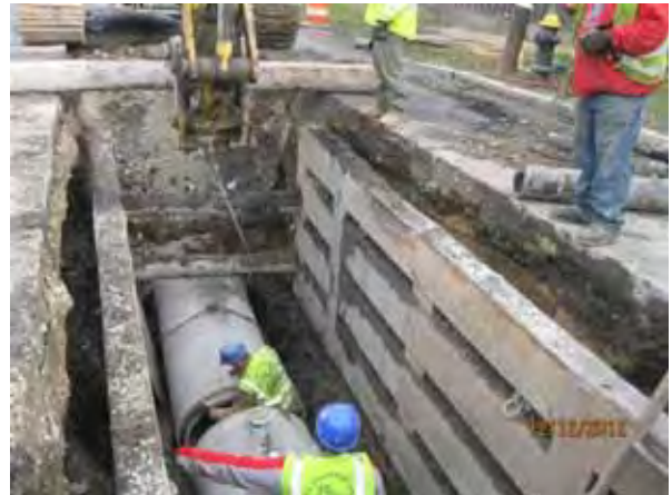
Installation of 36-inch drain on E Street Reserved Channel Sewer Separation Contract 4
