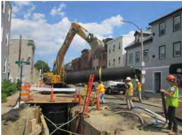
Installation of 42-inch drain on East Second Street Reserved Channel Sewer Separation Contract 3B
