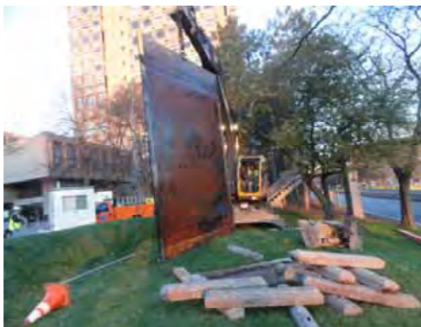
Removal of the overflow plate in Outfall MWR010 completed the Brookline Sewer Separation project
