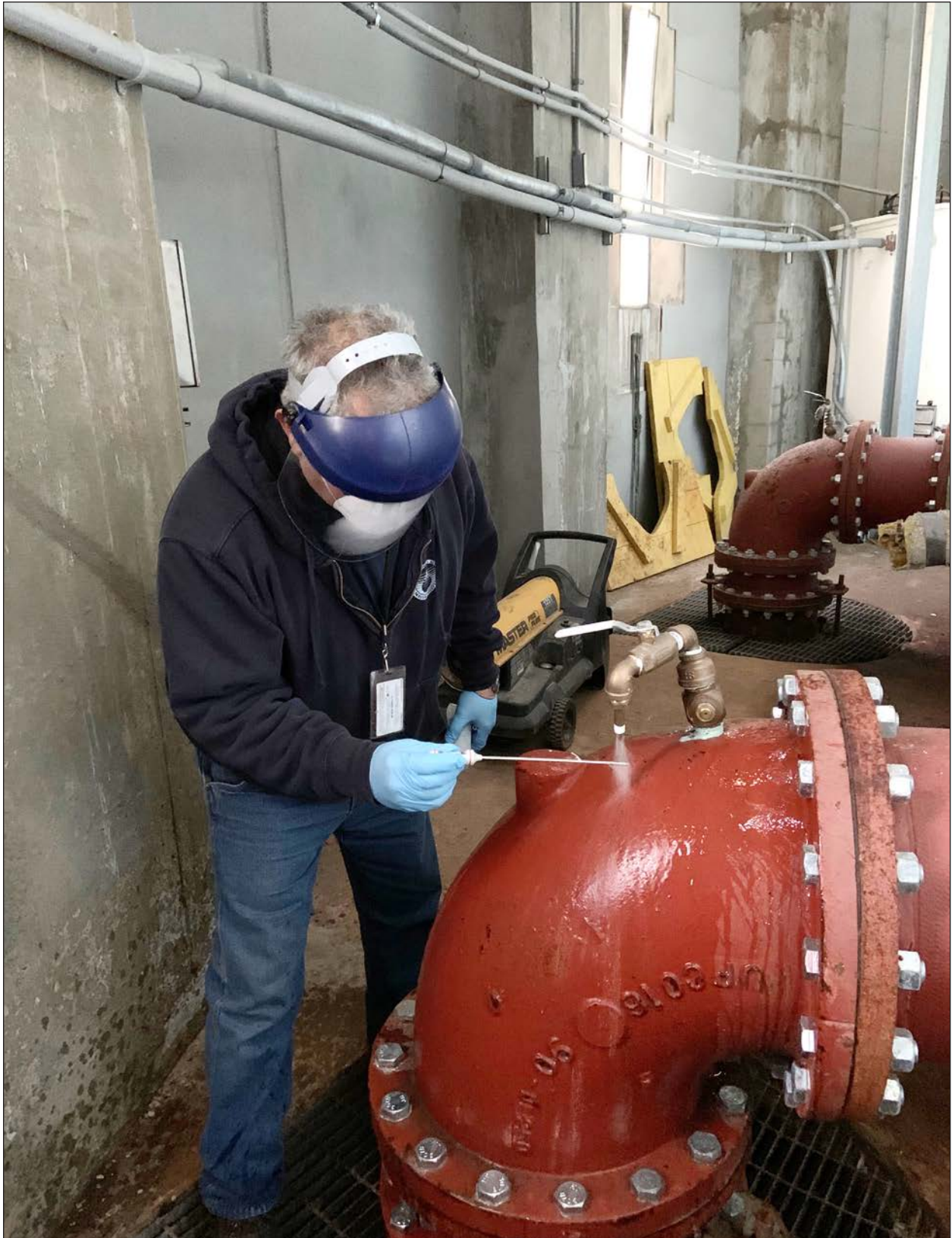
Temperature reading at Park Circle tank in Arlington
