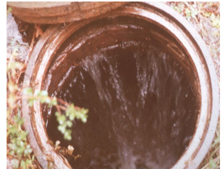
Inflow into a Manhole
