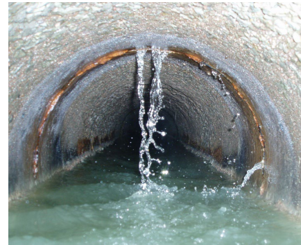
Infiltration in a Sanitary Sewer
