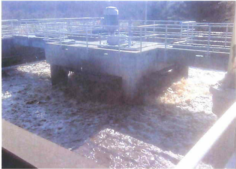
Aerator Assembly in Basin 5
