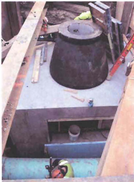
Figure 3: Forms being removed from Special Drain Manhole "A" at East First St. and I St.
