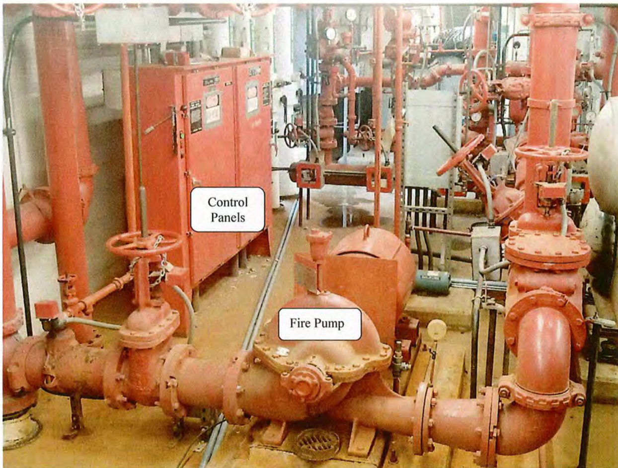
One of numerous fire pumps located throughout Deer Island
