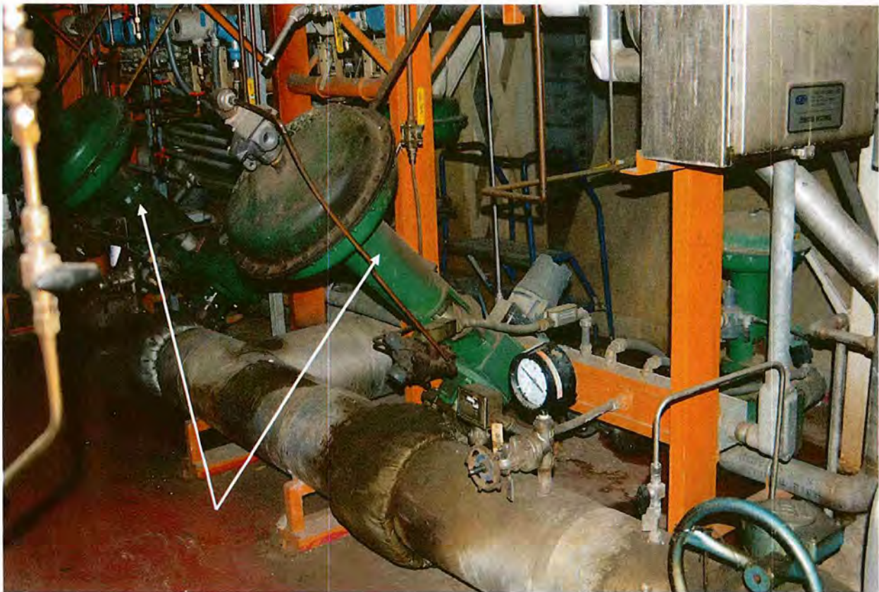
Digester control valves and actuators – a total of four; two for each boiler (shown is mid-level of boilers) will be replaced because of low-flow instability; the new valves will operate more accurately and efficiently, and with better range at low flows.
