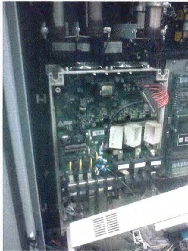
Variable frequency drive at Cosgrove required replacement due to overheating and damaged components
