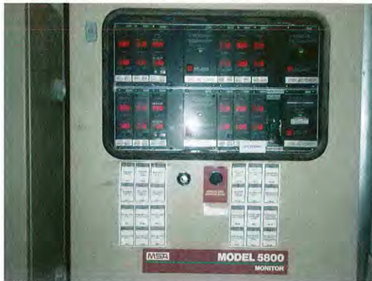
One of three gas monitoring control panels at the Nut Island Headworks
