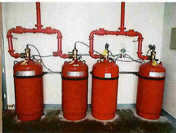
One Halon fire suppression set-up in the Administration/Laboratory Building
