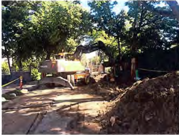
Contract 8B work has required extensive road closings in the Huron Avenue neighborhood
