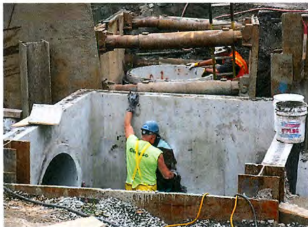
Drain Vault #1 at Vassal Lane and Standish Street, Contract 8A
