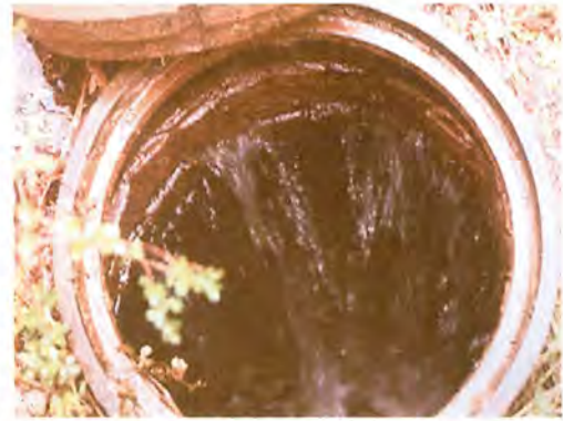
Inflow into a Manhole
