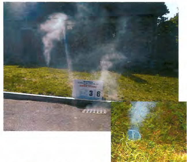
Smoke Testing of Sewer Confirms Catch Basin and Open Clean-Out are Inflow Sources
