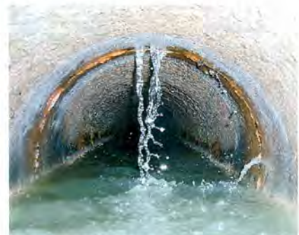
Infiltration in a Sanitary Sewer
