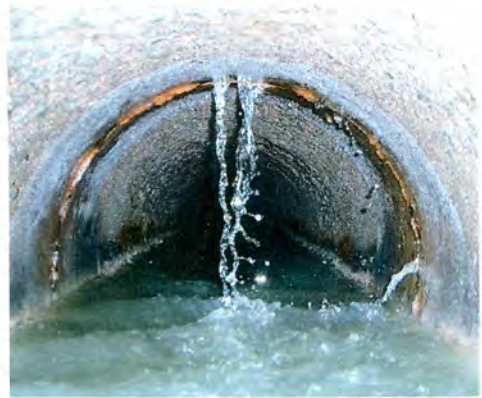
Infiltration in a Sanitary Sewer
