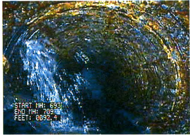
Infiltration Source Identified by Sewer TV Inspection
