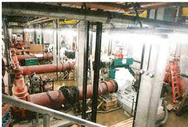
Pump Station Interior
