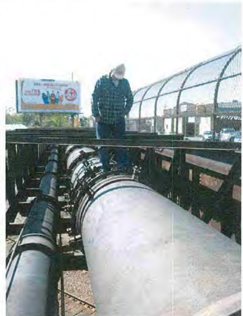
Somerville's 20-Inch and MWRA's 48-Inch Pipeline on Utility Bridge
