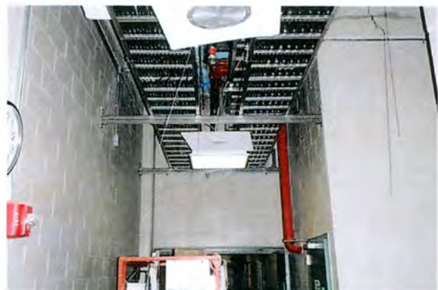
New Cable Trays in First Floor Hallway
