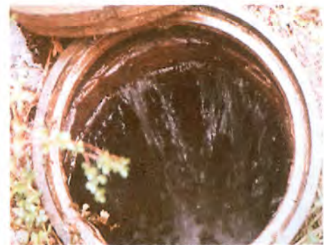
Inflow into a Manhole
