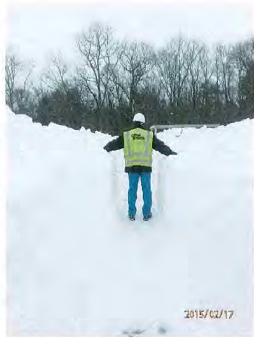
Substantial Snow Depth on the Roof of the Storage Tank in February 2015
