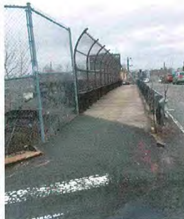
Traffic and Foot Bridge will not be Replaced
