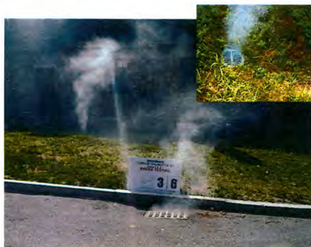
Smoke Testing of Sewer Confirms Catch Basin and Open Service Connection Clean-Out are Inflow Sources
