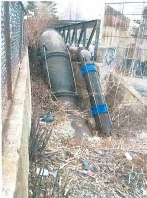
MWRA Pipe and Somerville Pipe Rising from Underground and Across Bridge
