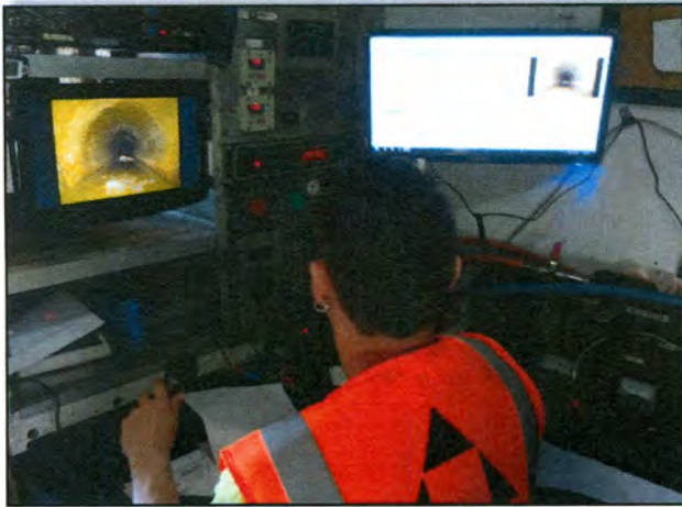
Sewer TV Inspection
