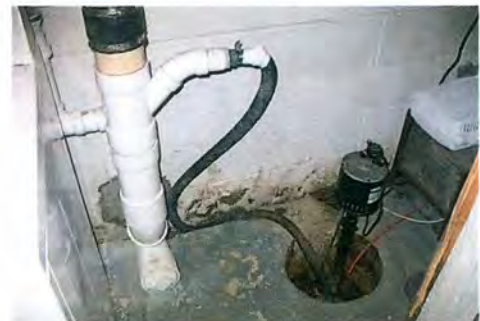
Private Inflow from a Sump Pump
