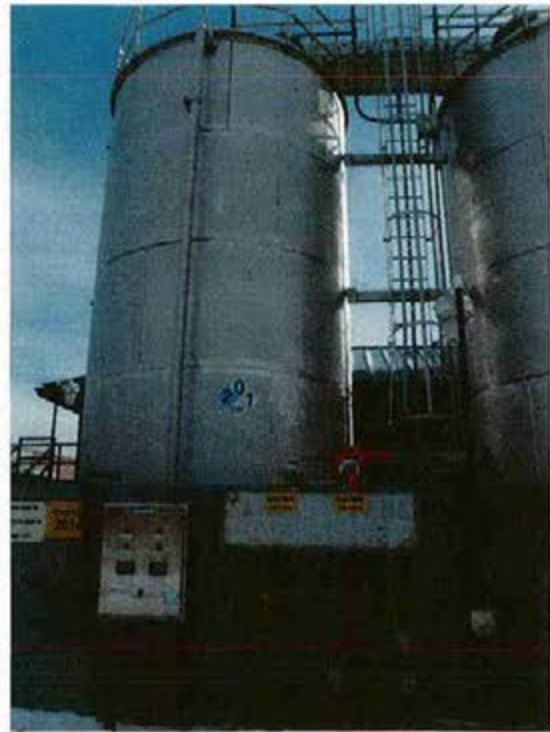
North System Storage Tanks
