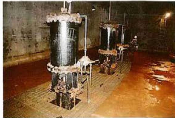
Shaft 7 Hydraulic Valve Operators
