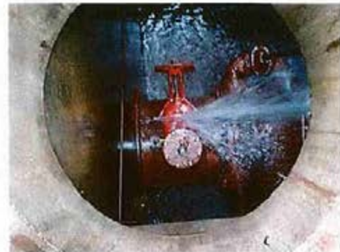
Leaking valve bonnet in 2012
