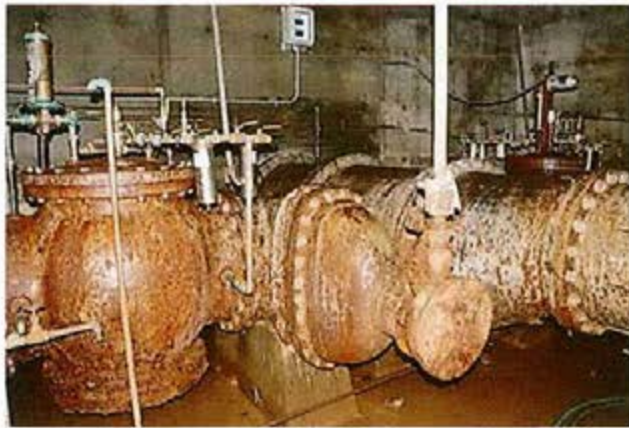
Shaft 8 Isolation valves and PRVs
