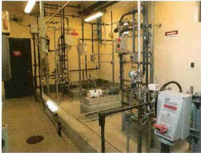
South System Hydrogen Peroxide Pump Room
