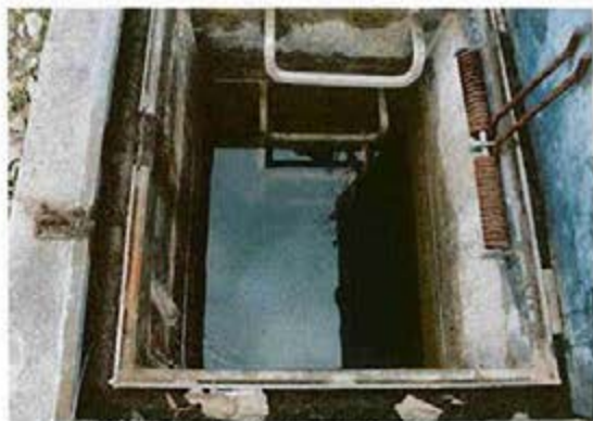
Ground water in top of Shaft Chamber
