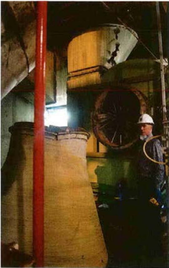
Scrubber #4 Exhaust Fan Inlet Damage
