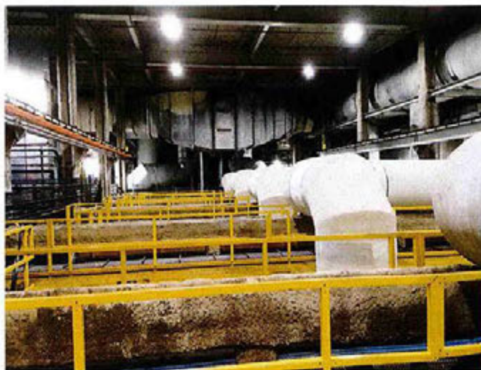
Figure 1 – Cleaned OC Room
