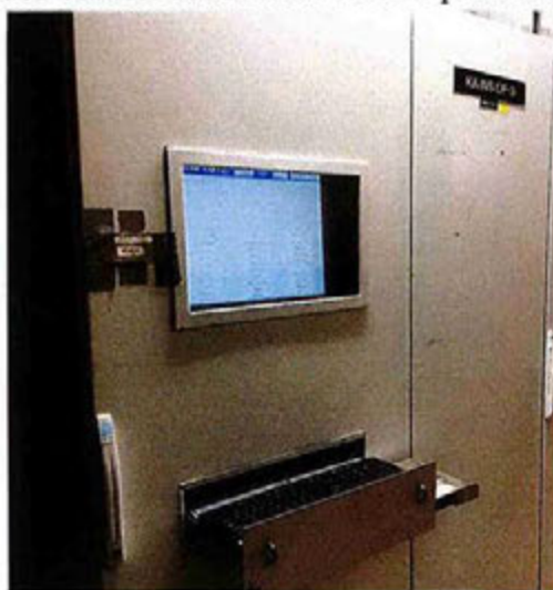
Figure 3 – SCADA Panel Energized
