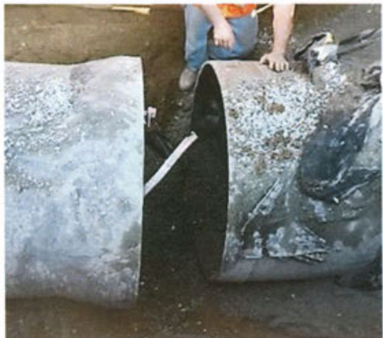
Figure 2. First Failed HP LOK joint.
