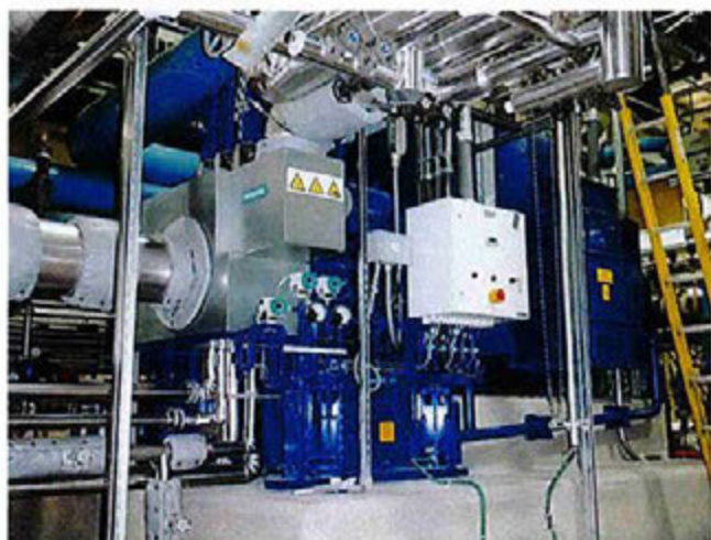
1.2-Megawatt Back-Pressure Steam Turbine Generator
