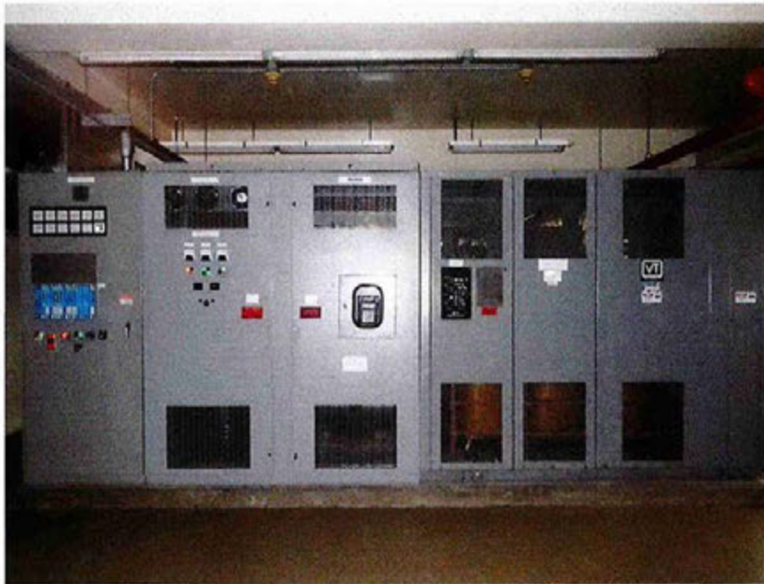
Raw Wastewater Pump Variable Frequency Drive (VFD)
