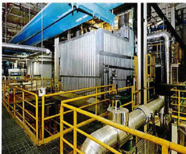
Two High-Pressure Steam Boilers
