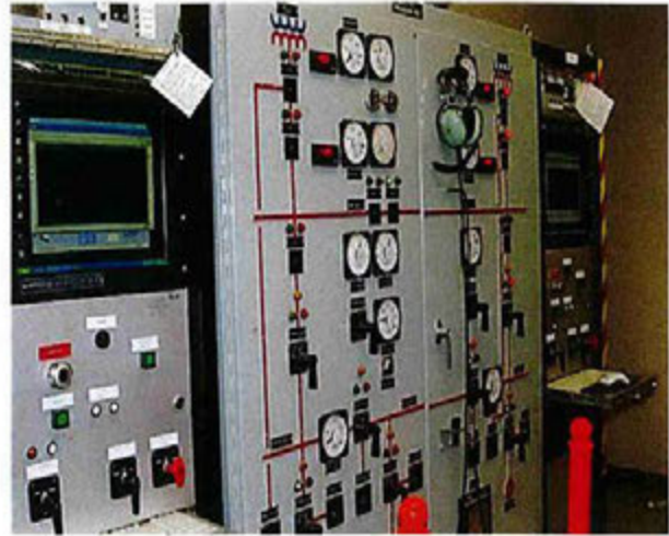
One set of control panels
