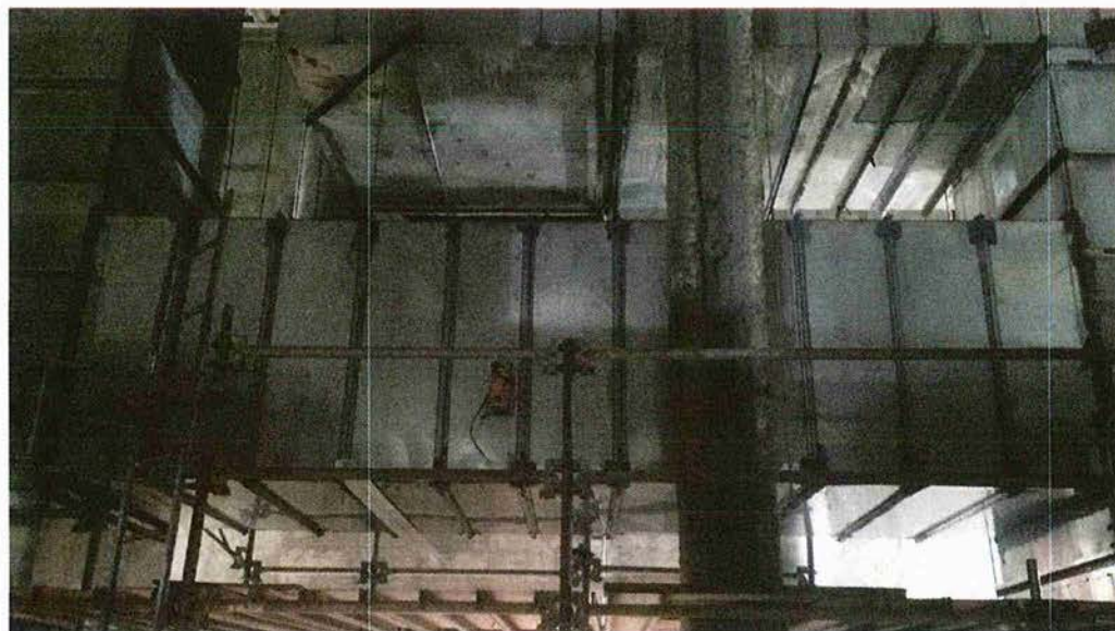
Interconnection Ductwork and Dampers between Wet Scrubbers 2 and 3
