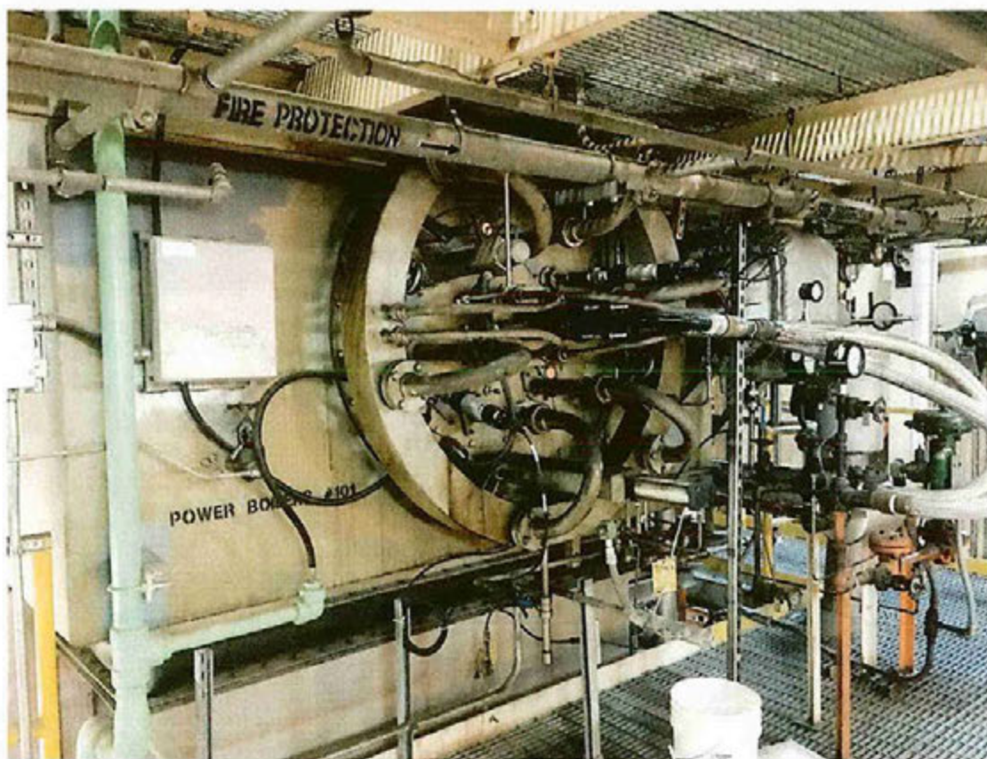
High Pressure Boiler (1 of 2)
