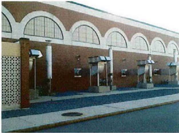
Air Compressor Building with Air Intake Ducts
