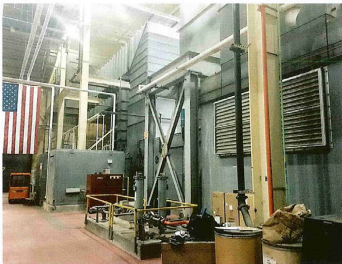
Combustion Turbine Generator (1 of 2)
