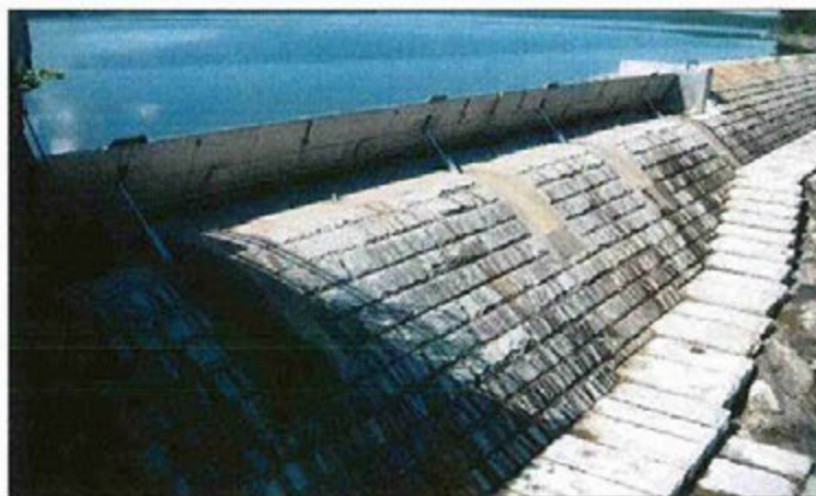
Figure 4. Wachusett Spillway Crest Gate
