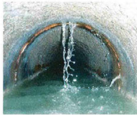
Infiltration in a Sanitary Sewer
