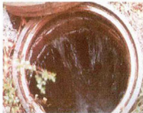
Inflow into a Manhole
