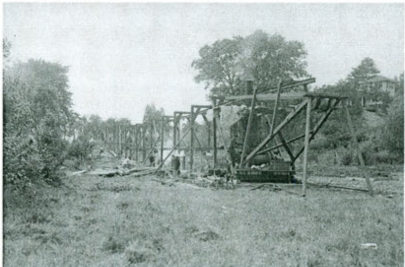
Construction of a section of the Reading Extension Sewer (circa. 1919) along Prospect Street near the Stoneham/Wakefield town line.
