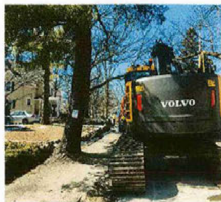
Tree to be removed on Oak Street
