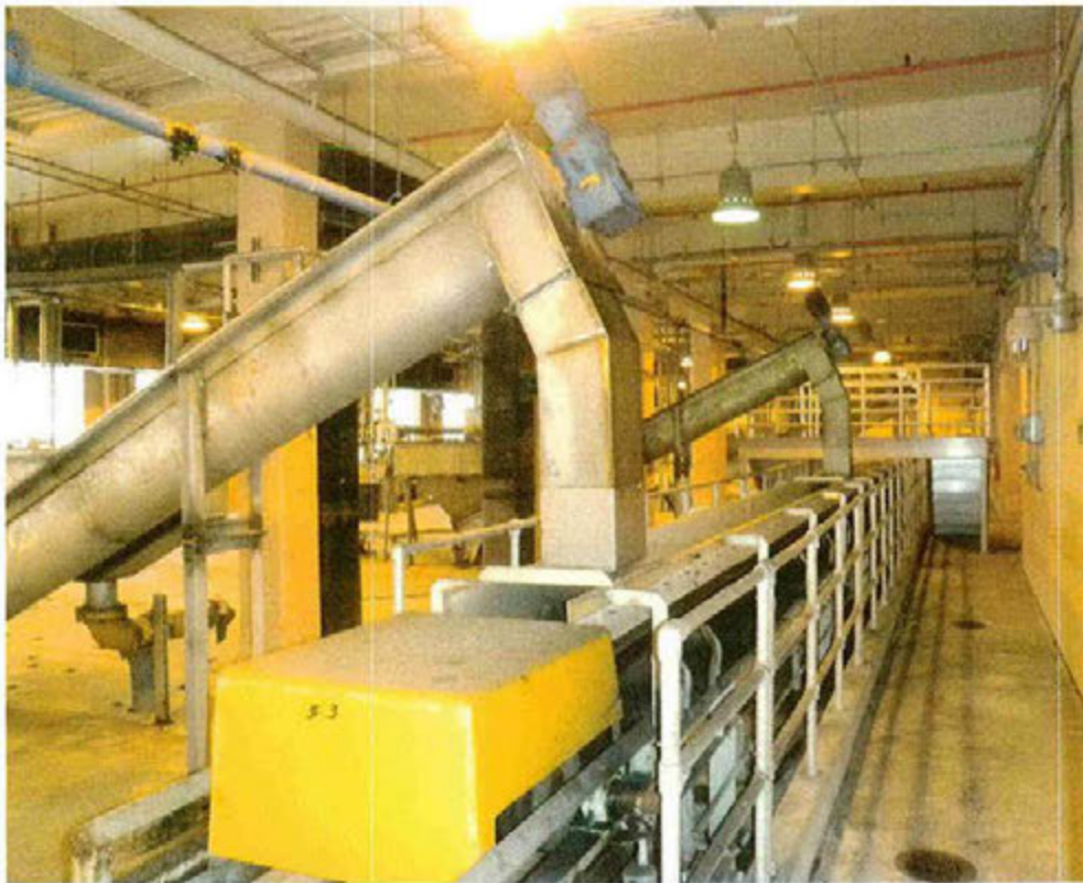
Shown are Two of 16 Grit Classifiers in the Grit Facility that Deposit the Grit onto the Conveyor
