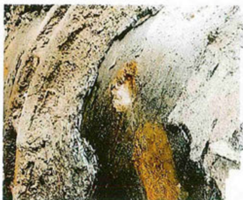
Pipe showing corrosion
