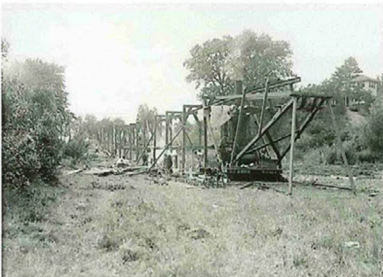
Construction of a section of the Reading Extension Sewer (circa. 1919) along Prospect Street near the Stoneham/Wakefield town line.
