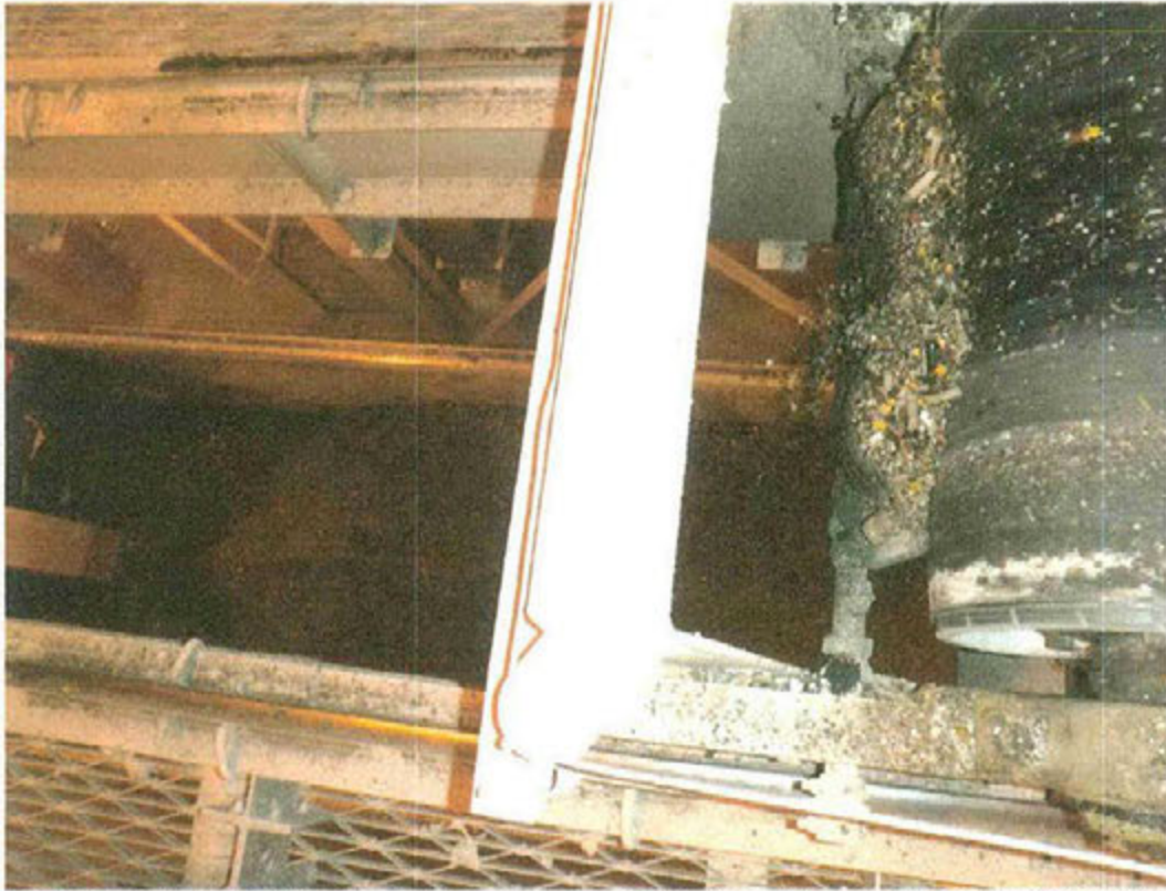
Grit Being Removed by the Belt Scraper and Dropping into Trailer Below. Conveyor Operates 24/7 and the Entire Belt Assembly Moves Fore and Aft to Distribute the Grit Evenly in the Trailer.
