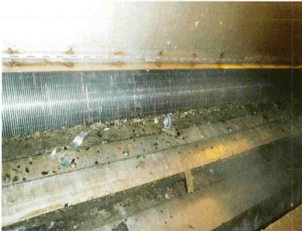
One of Deer Island's Four Primary Scum Screens for Removing Inorganic, Largely Indigestible Material from the Wastewater Prior to Gravity Thickening
