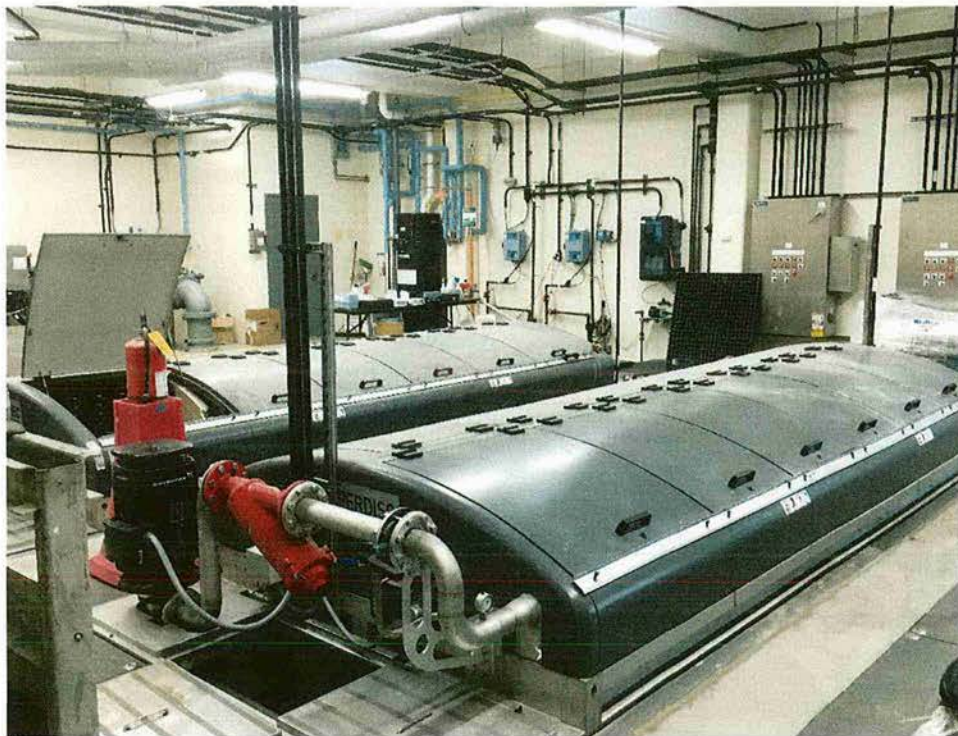
Disc Filter Process Equipment in New Phosphorus Reduction Facility
