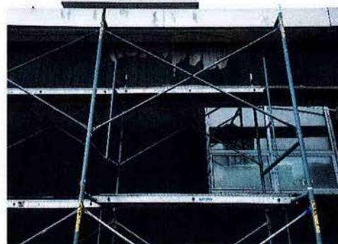
Black tar paper on exterior building panels containing asbestos
