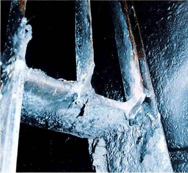
Broken and Corroded Bars
