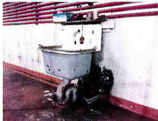
Janitor sink with "S" trap not properly vented
