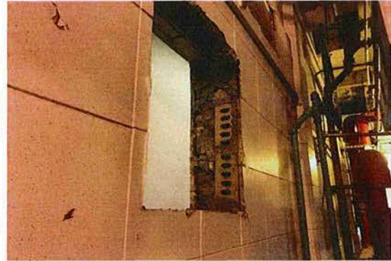
Interior Walls Constructed of 4-inch CMU Instead of 8-inch
