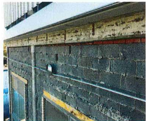
CMU Not Properly Secured to Building Structure
