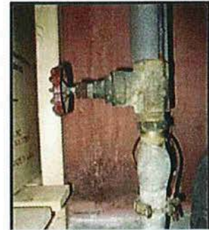
Lead Service Line Entering Basement
