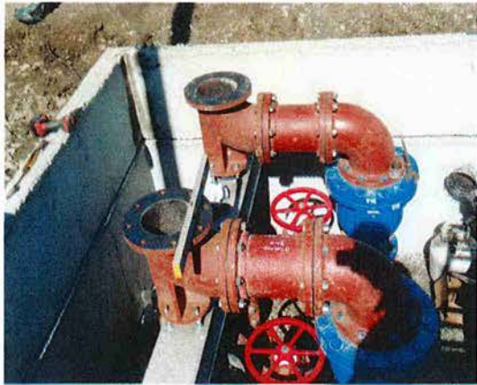
Air Release valve piping
