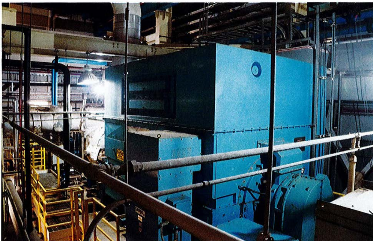
Figure 2 - Steam Turbine Generator
