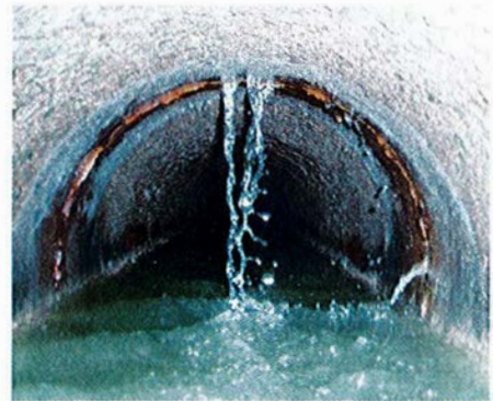
Infiltration into a Sanitary Sewer
