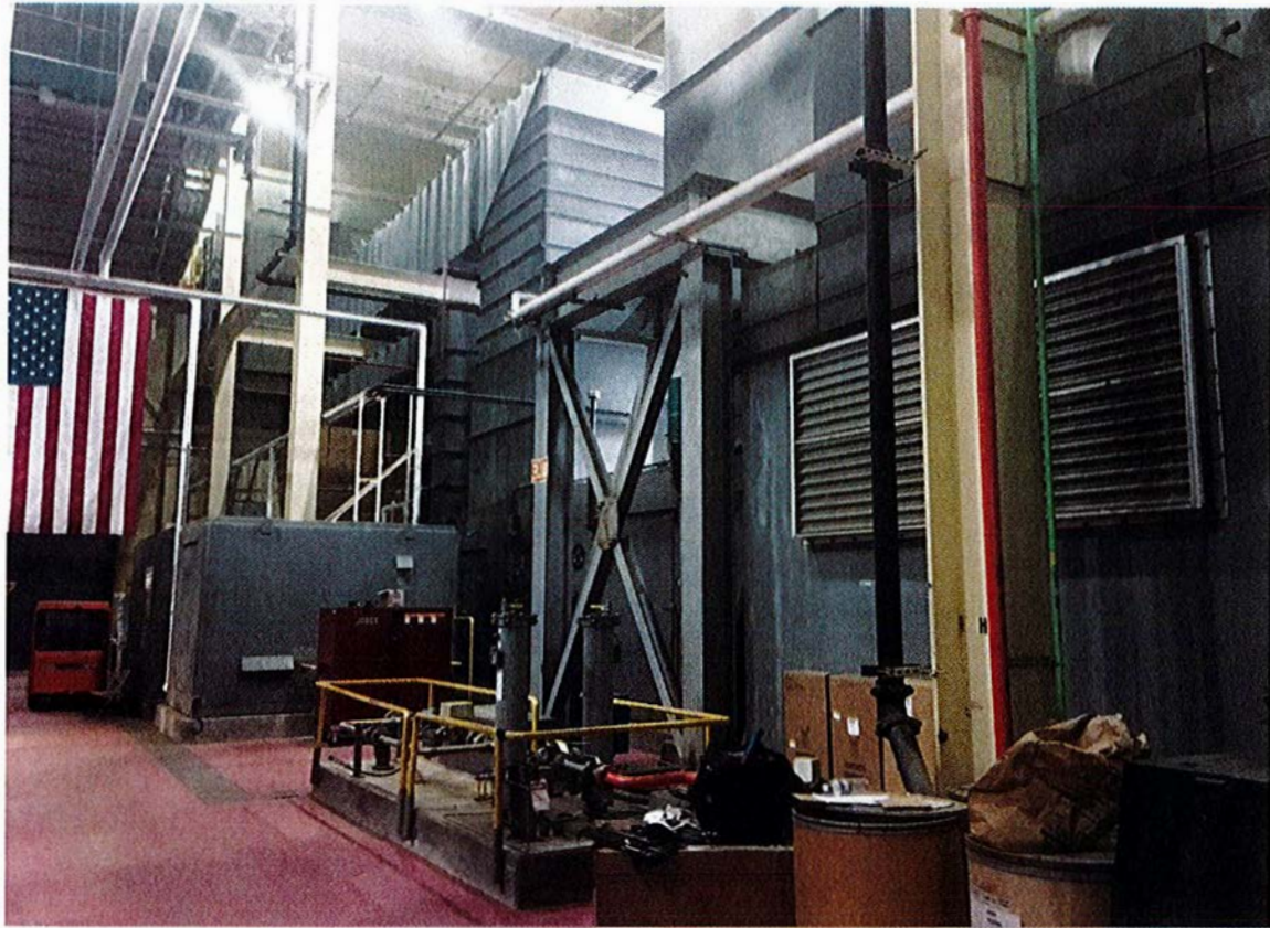
Figure 1 - Combustion Turbine Generator
