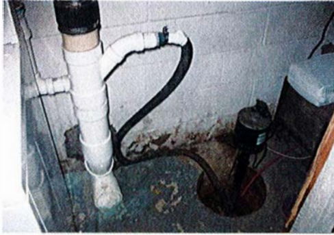
Private Source Inflow from a Sump Pump
