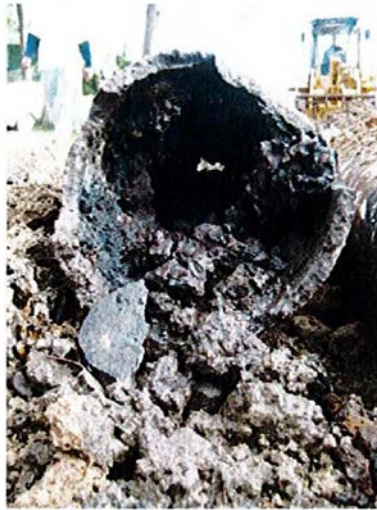
Old Unlined Cast Iron Water Main Pipe
