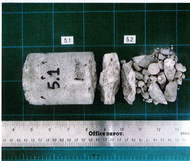
Core Sample from Foundation Showing Deteriorated Concrete
