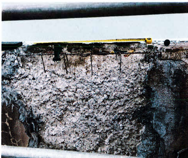
Concrete Foundation at Turkey Hill Tank showing existing rebar and extensive delamination
