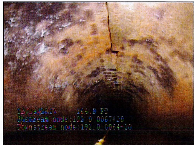
Figure 3: Crown crack and missing brick in Section 192
