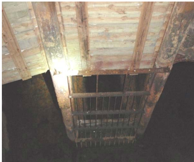
Wooden Stop Plank Gates
