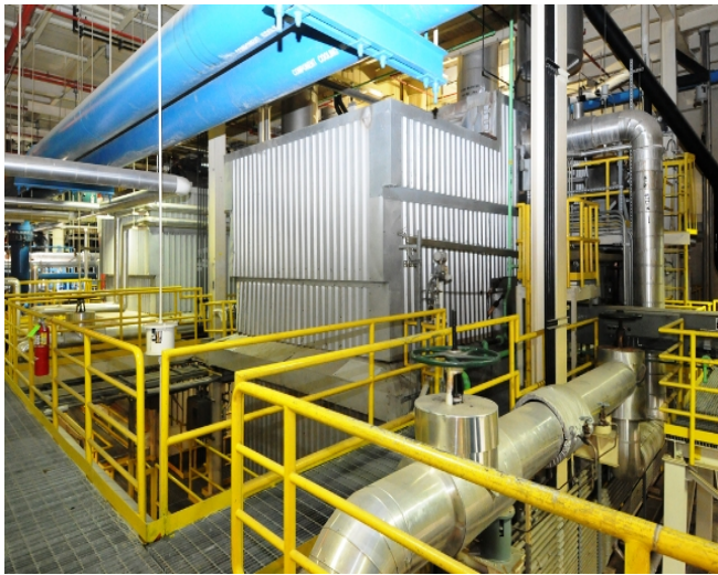
Figure 1: Two High - Pressure Steam Boilers at Deer Island
