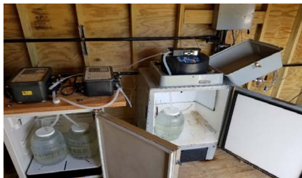
Figure 3. Autosamplers at the Clinton Wastewater Treatment Plant
