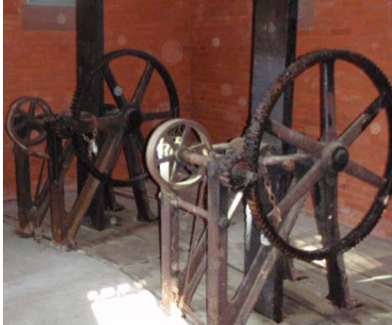
Gate's Rack and Pinion Lifting System
