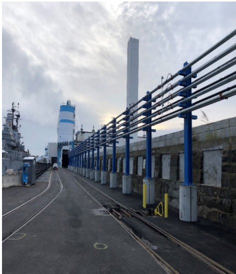
Figure 3 Pipe Support Posts
