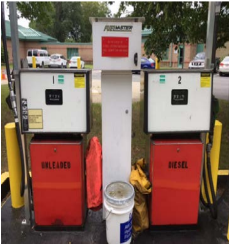
Figure 3- Southborough Fuel Pumps
