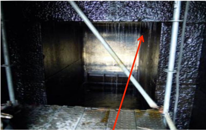
Leakage through stone joints
