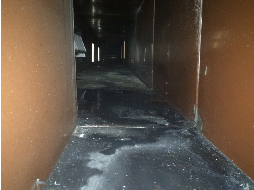
Soot in HVAC Ductwork
