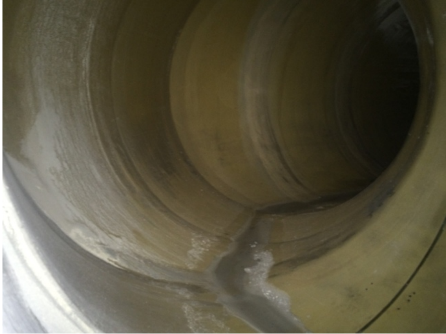
Dust in Odor Control Ductwork
