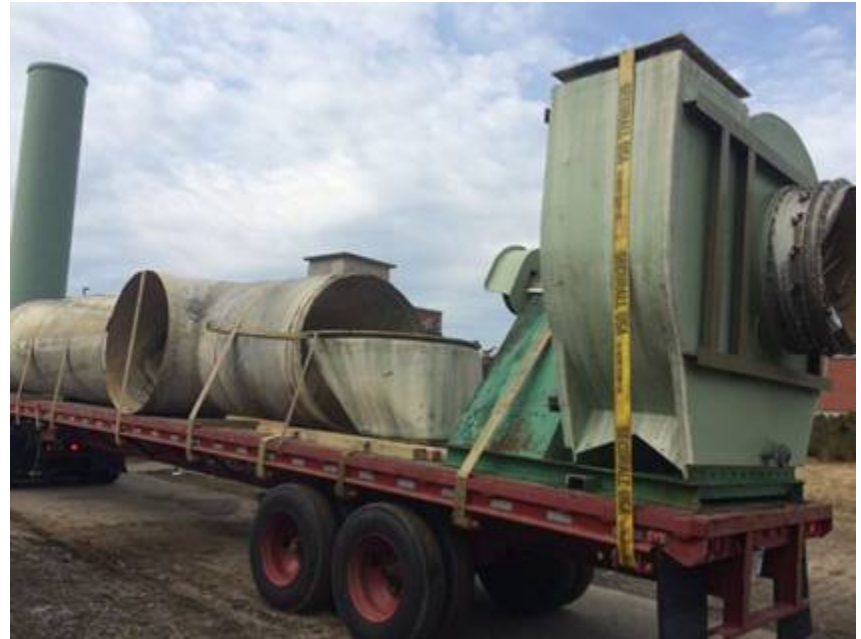
Removed Failed Fan and Ducting
