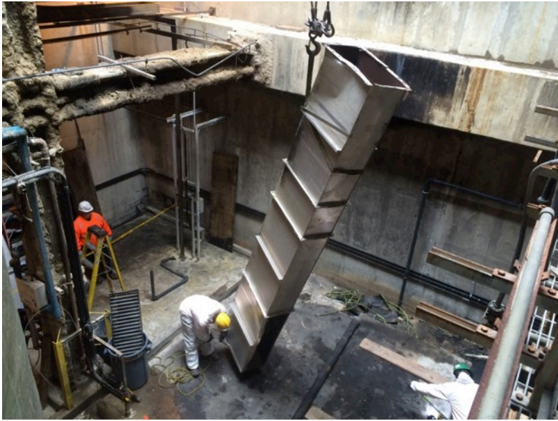
Failed/Burnt HVAC Duct Removal
