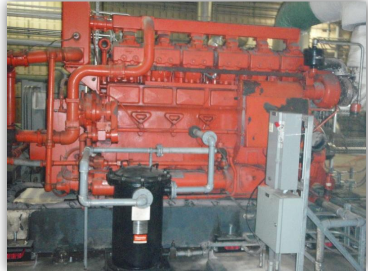
Diesel Engine Powering Wet Weather Pump
