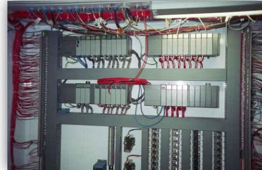
Programmable Logic Controller (PLC)
