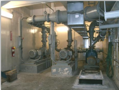
Dry Weather and Dewatering Pumps
