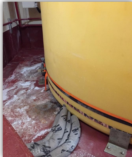
Leaking Chemical Tank
