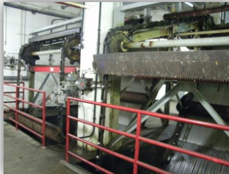
Mechanical Bar Screens
