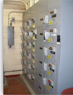
Motor Control Center
