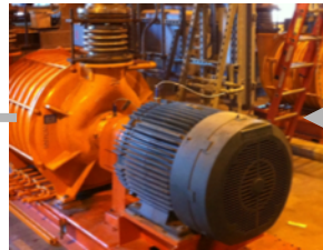
Biogas Booster Blowers
