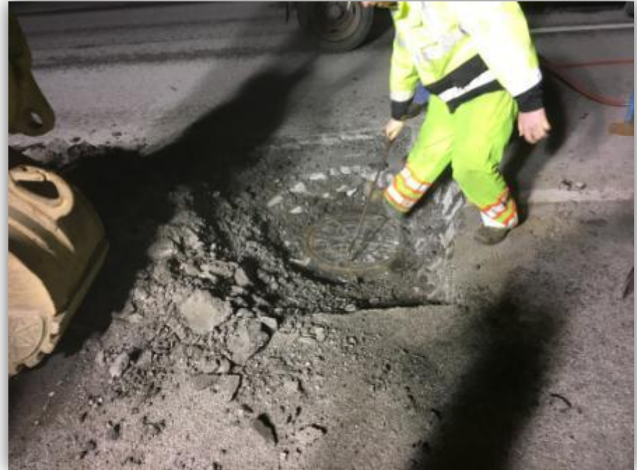
Buried manhole cover found 4/2, 10:45 P.M.
