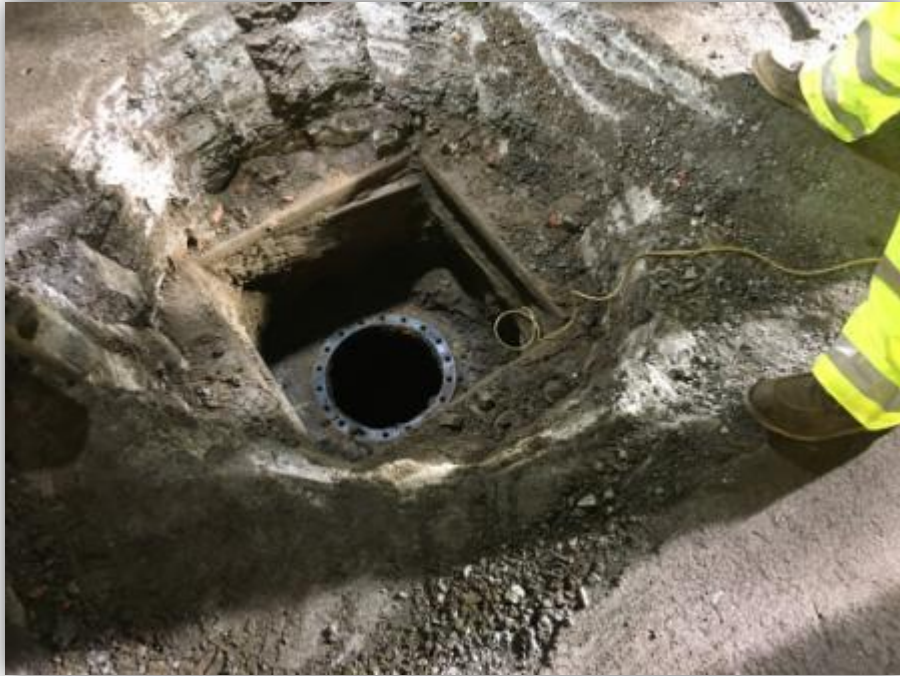
Top of Flange without A.R.V 4/3, 12:05 A.M.
