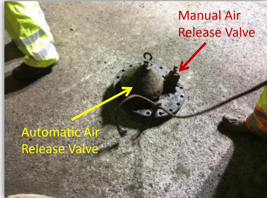
Air Release Valve Assembly (mounted on flanged plate)
