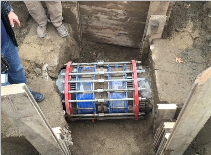
Joint excavated after leak
