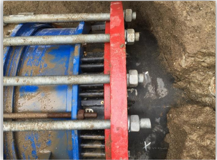
Fusion location of flex restraints on east side after 1 st repair
