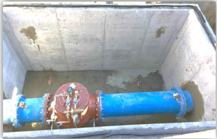
Town of Reading Valve Vault
