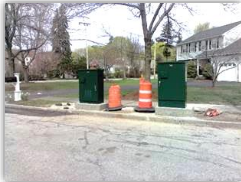
Above Ground Meter Cabinets
