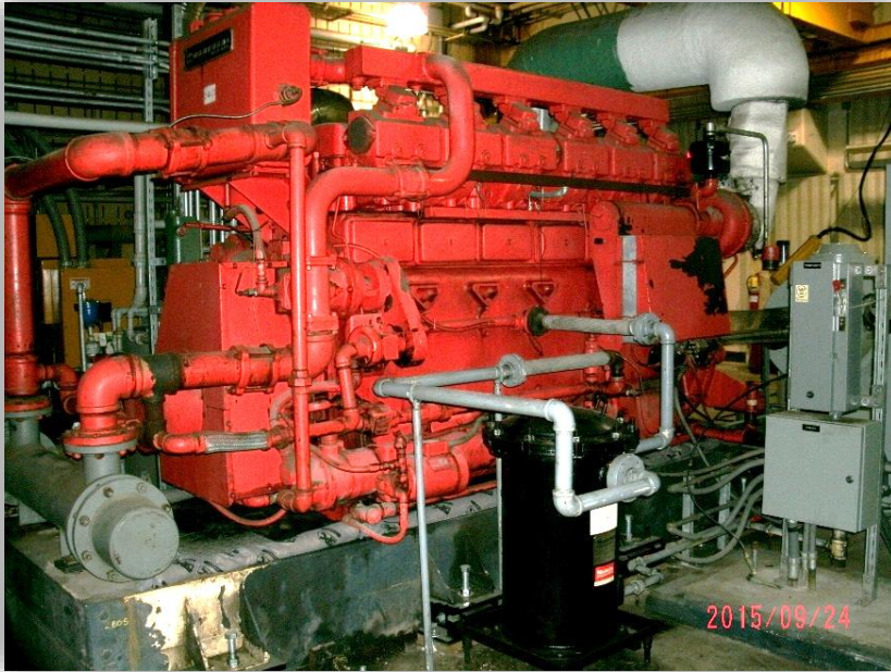
Storm Pump Engine to be Replaced
