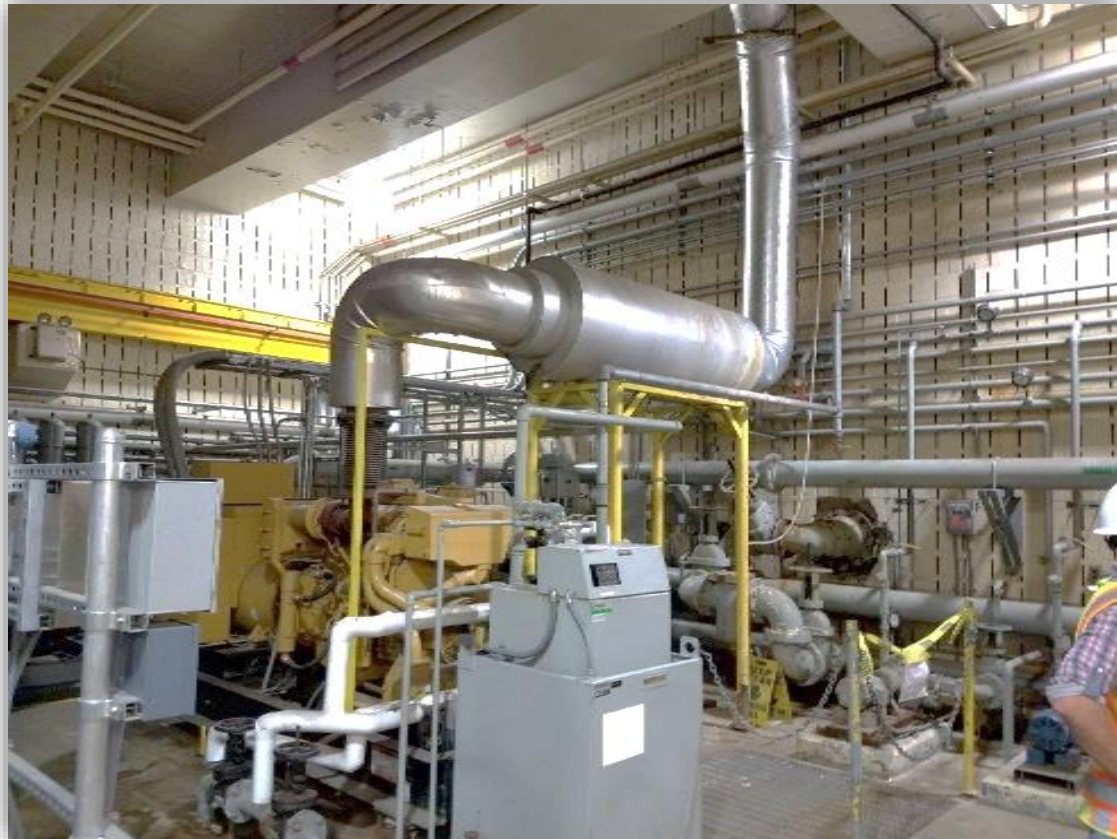
Generator to be Replaced
