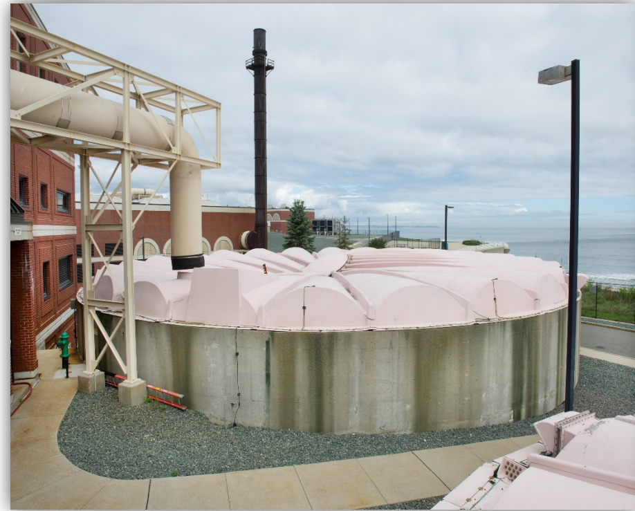
Collapsed Fiberglass Dome Cover
