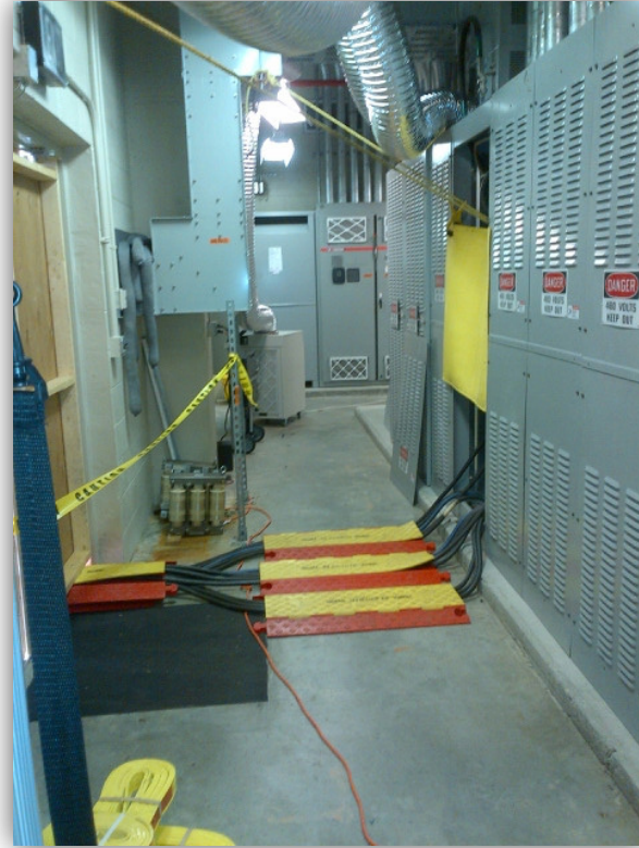
Direct Wiring to Switchgear
