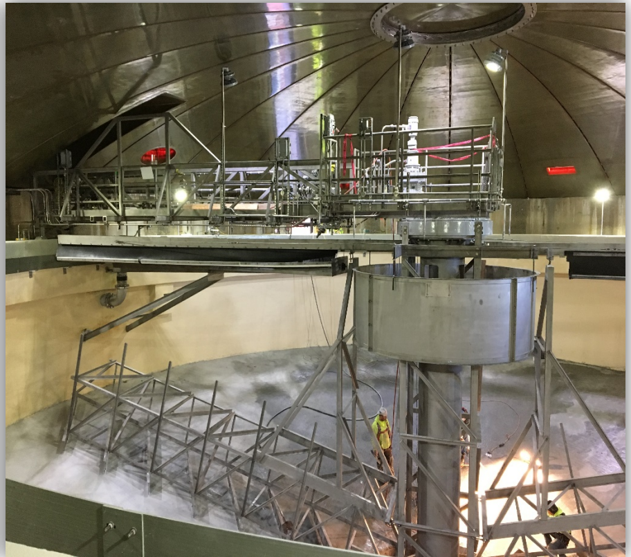
Interior of GT
