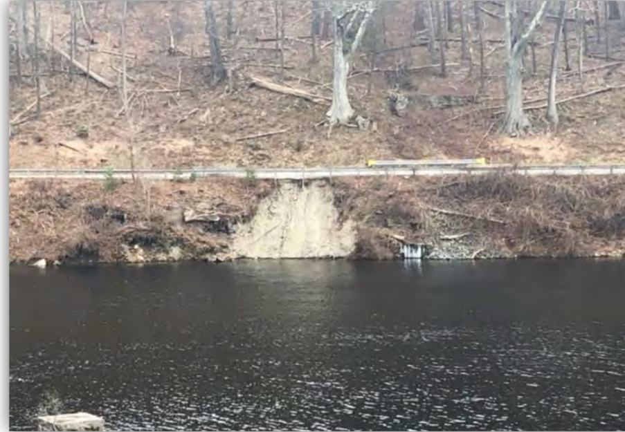
November 2018 River Road Landslide
