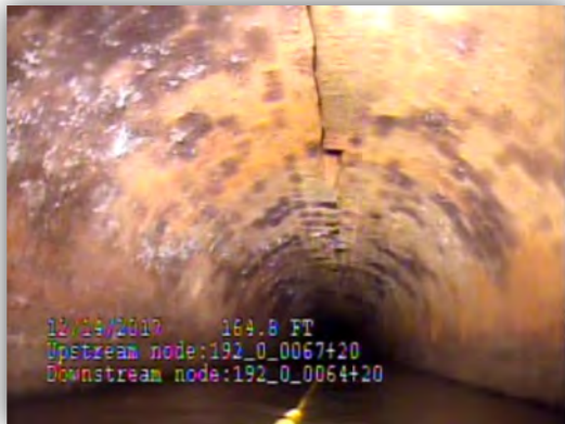
Section 192 Crown Crack and Missing Brick
