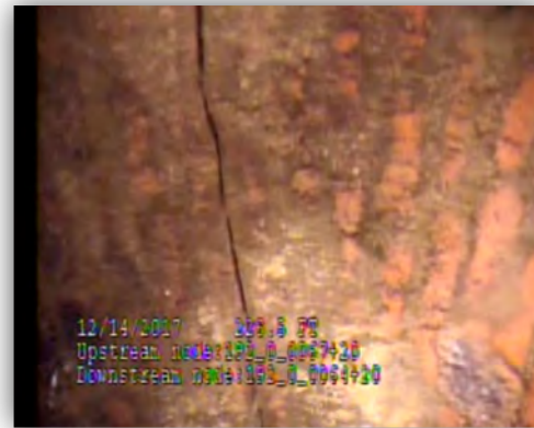
Section 192 Crown Crack
