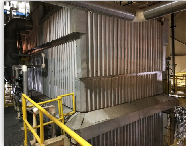
Existing Steam Boiler
