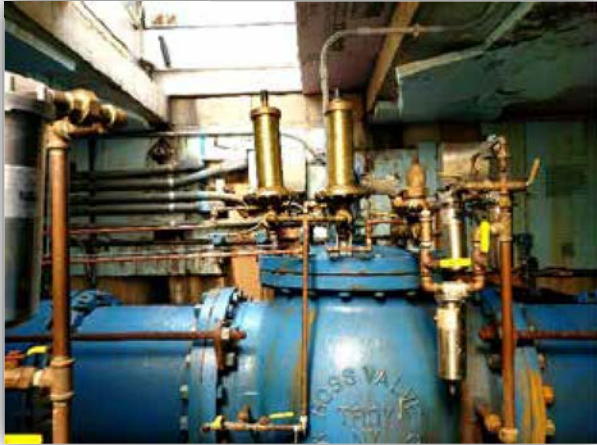
W14 Nonantum Road Vault and PRV (existing)
