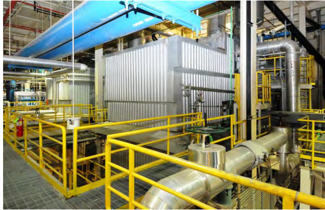
High Pressure Boilers
