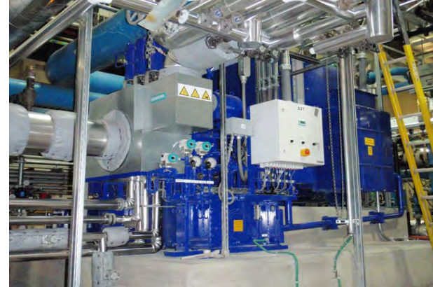
Back Pressure Steam Turbine Generator
