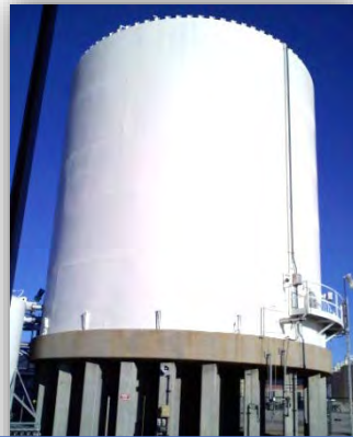
1,000 Ton Liquid Oxygen Storage
