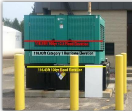
Chelsea Creek Screen House Backup Generator
