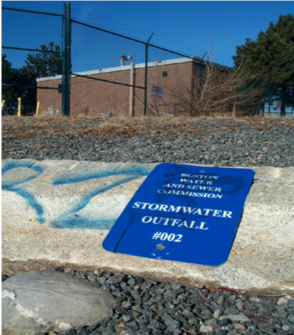
MWRA decommissioned its Constitution Beach CSO Facility after CSO flows were eliminated by BWSC sewer separation.
