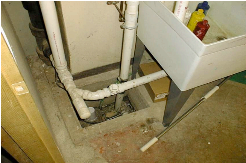
Sump Pump Inflow
