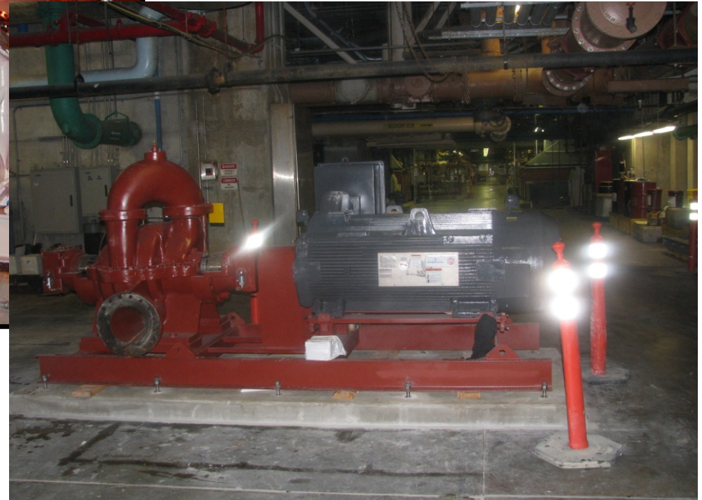
Sludge Pumping to NEFCO – Existing and Proposed
