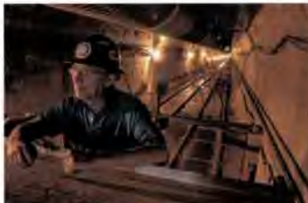
Operating machine Dick Pentecost removes the 2-mile railway system that diverts workers and sludge back and forth through the tunnel.
