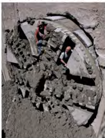
Tunnel workers Steve Chigg (left) and Patric Rusk emerged from underground yesterday about their 18-foot boring machine. For almost a year, the machine had been digging a tunnel for the Massachusetts Water Resources Authority's sewer and storm runoff project.
