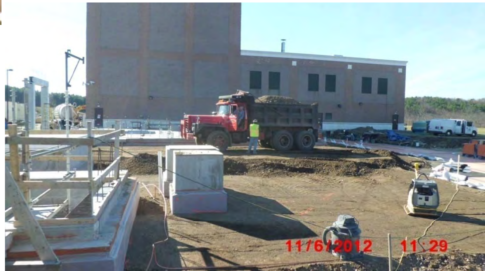
A Side Grounding Rods and Wiring
