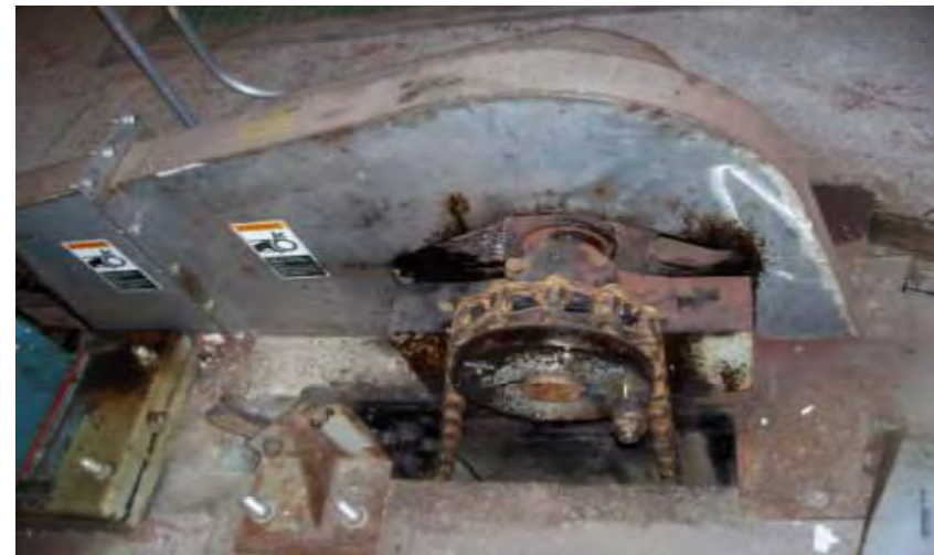
Grit Collector Drive
